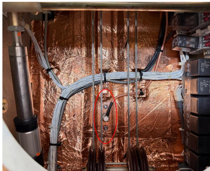
Figure 4: G1 Rear Seat Antenna Installed with Ground Plane
